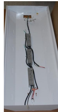
Figure 6: Example of a multiple LED Driver installation in a large gear tray. Drivers are inline and spaced 1"(25mm) apart.
