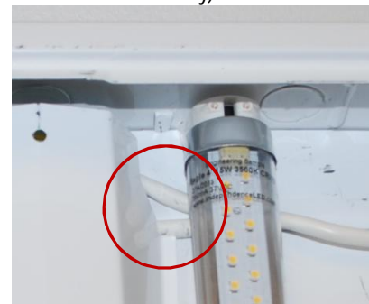
Figure 11: Routing of wires around edge of Wireway (circle)
